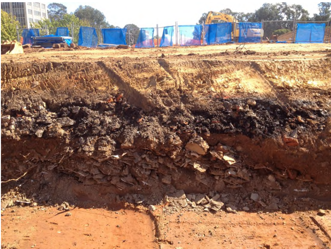
Photograph 6: Example building/demolition rubble with ACM in soil.
