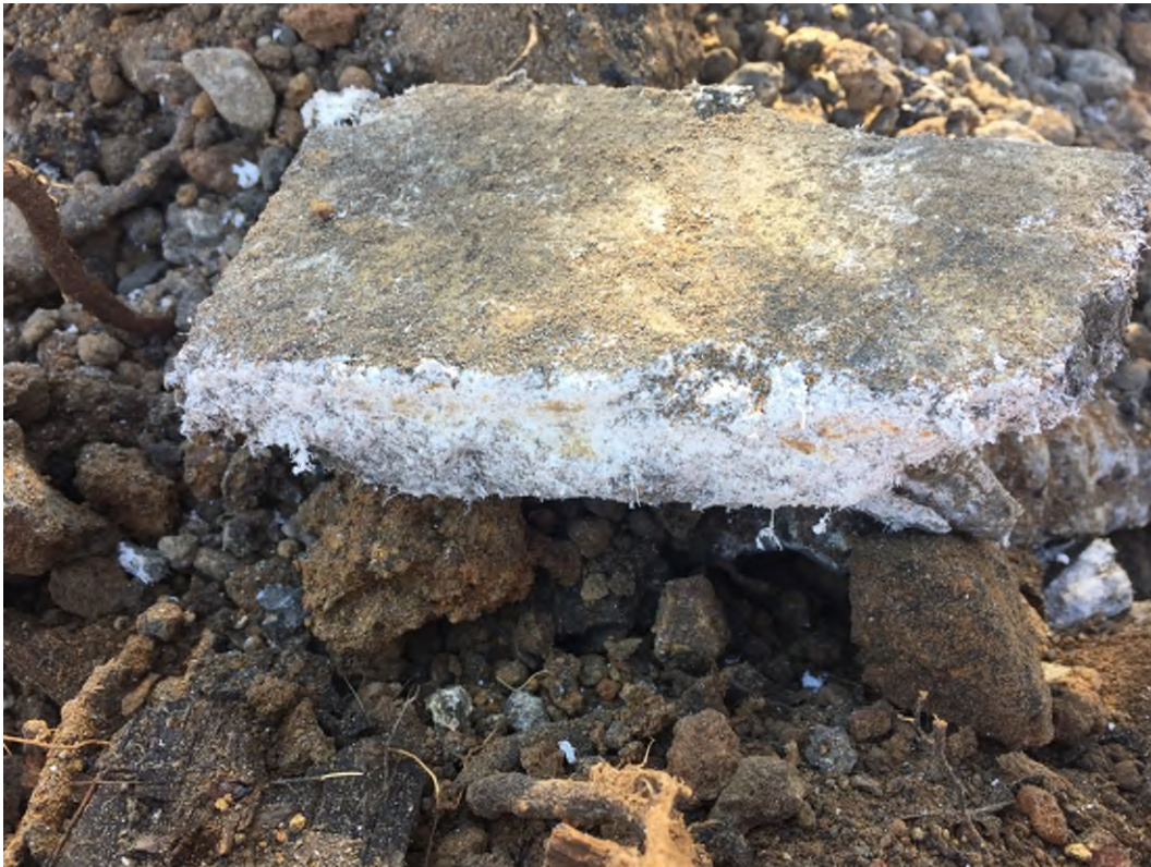
Photograph 9: Example close up of friable ACM insulation lagging in soil.
