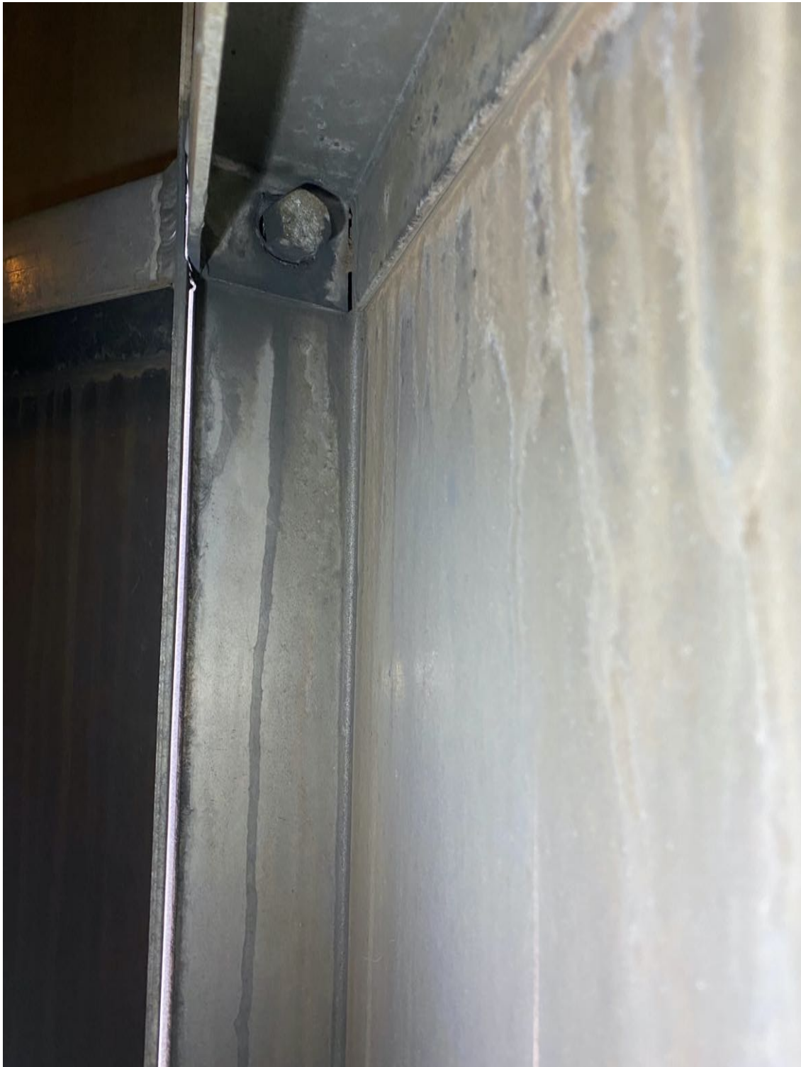
Example of wear and staining on a bolt on the side of a panel.
