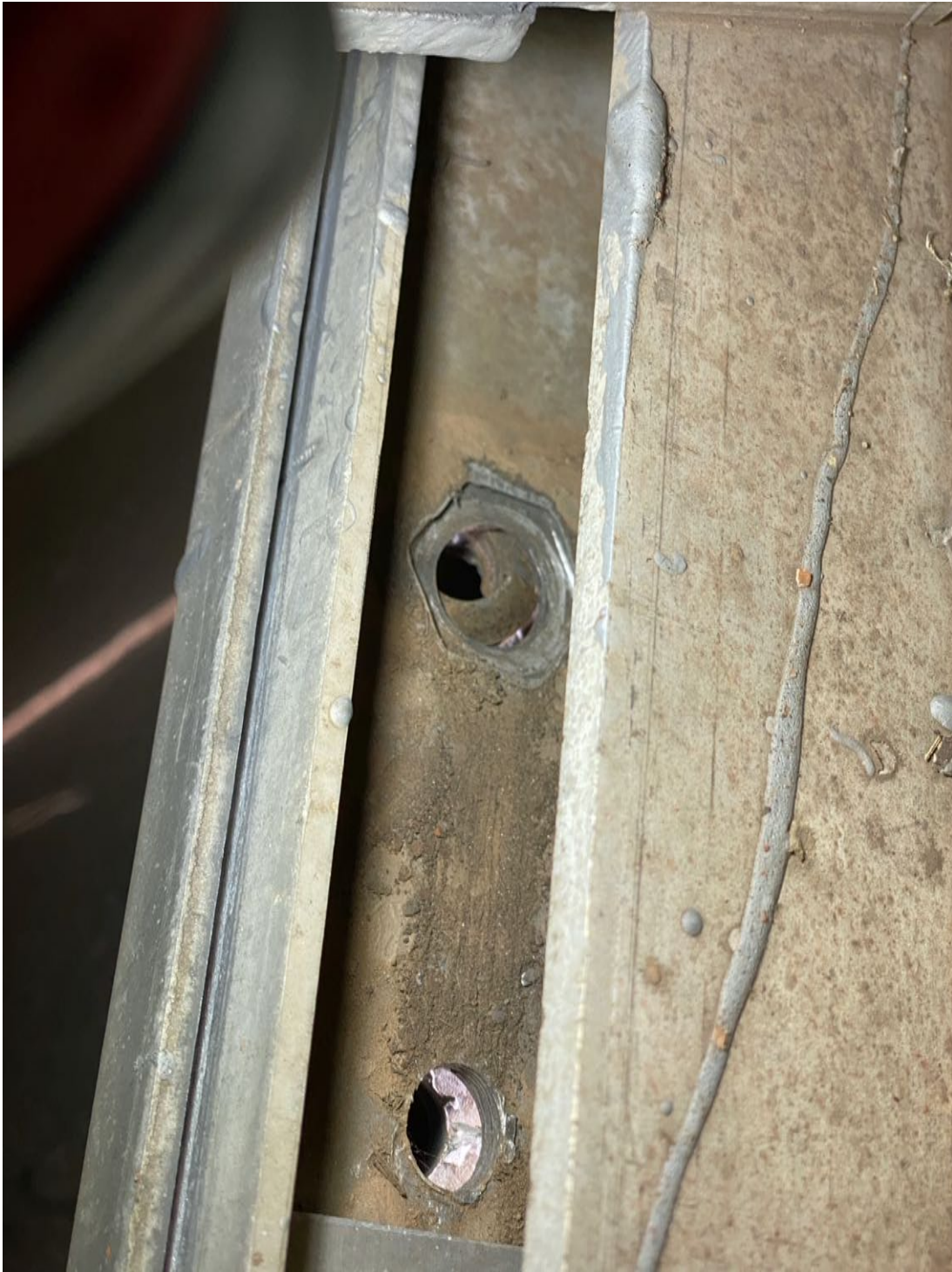
Example of abrasive wear to the fixing holes on the bottom of a panel, also note, fixings are missing.
