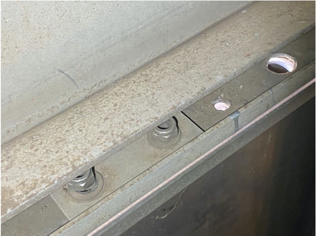
Example of bolts that have dropped out of nylock nuts leaving panels unconnected.
