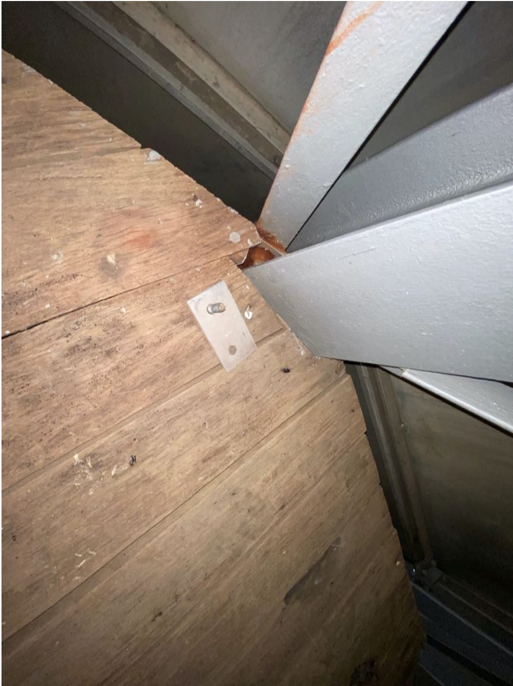
Example of red staining indicative of movement and bolts/plates fallen off the panels.
