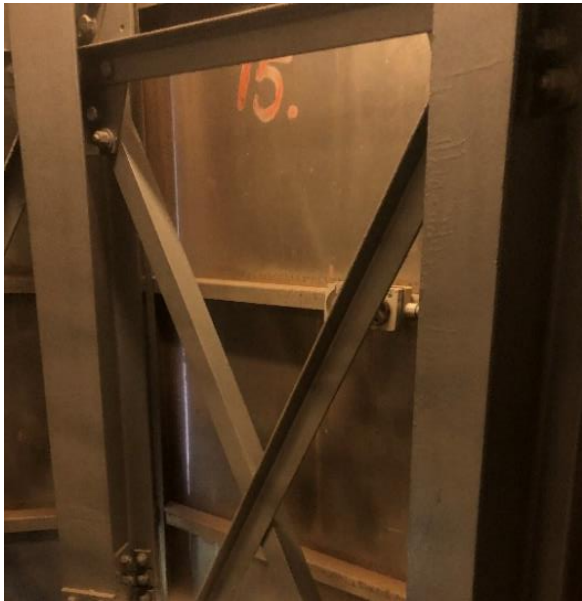
Figure 3.15 View of structural steel framework and aluminium panelling with the level number painted on the inside of the aluminium panel.
