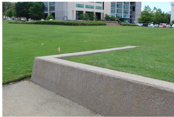
Figure 3.5 Exposed aggregate retaining wall that partly defines the northeastern boundary of Blamey Square.
