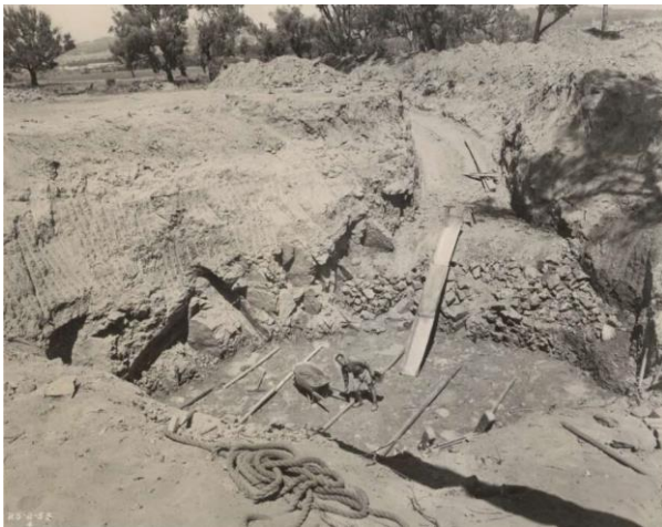
Figure 2.2 Excavation for the foundations of the column, February 1953. (Source: NLA, Bib ID 3665429)
