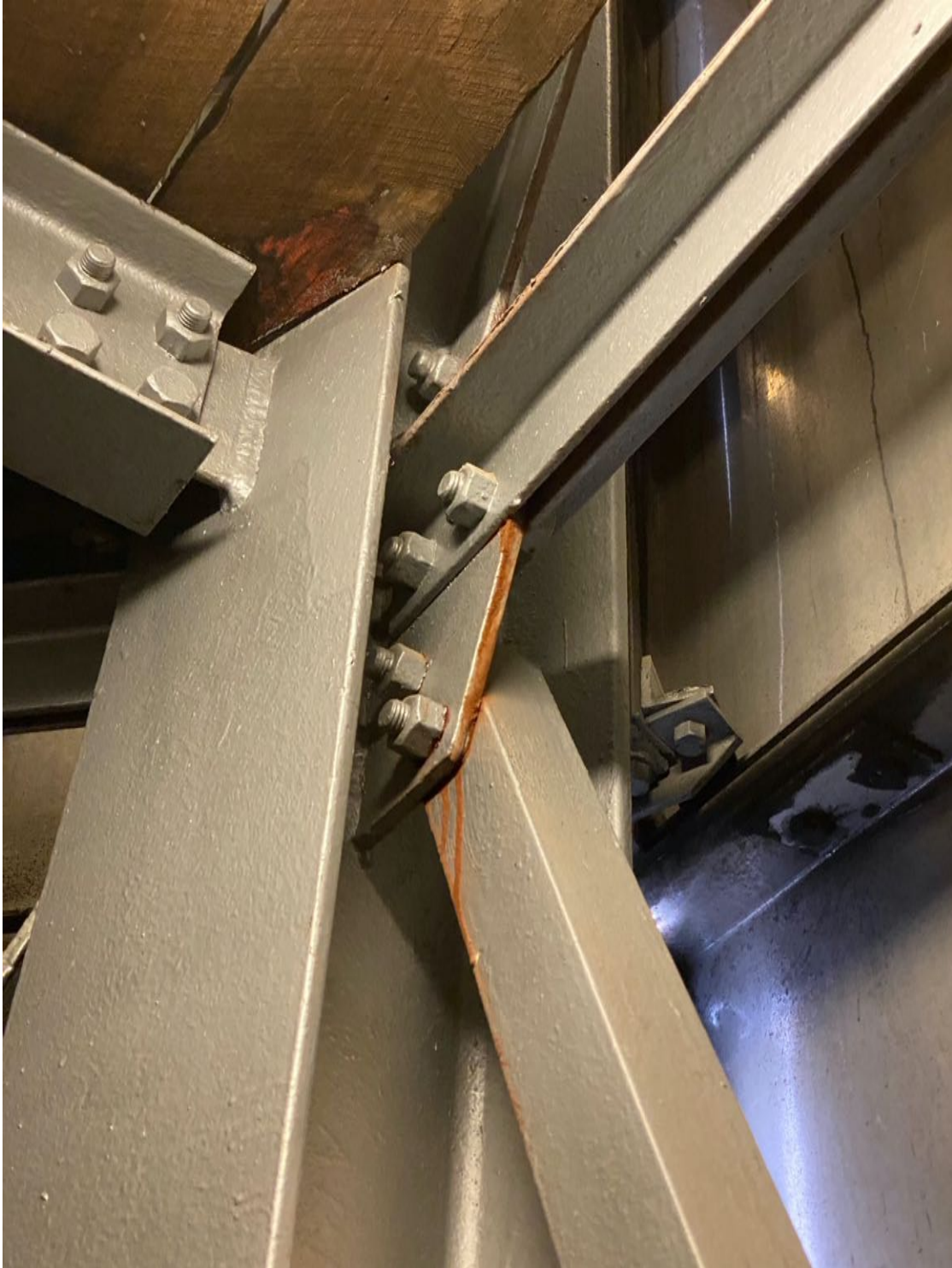
Example of red staining indicative of some movement in the structural frame.
