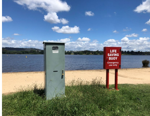
Figure 6: Electrical Services box and Life Buoy Enclosure
