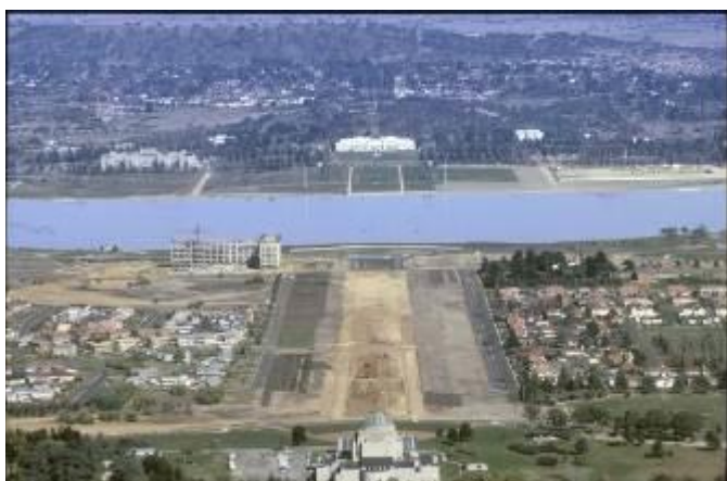
Figure 89. Earthworks showing both carriageways of Anzac Parade, Canberra, photo by Richard Clough, c1962
