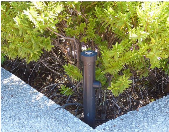
Figure 120. Spray risers blocked by plants
