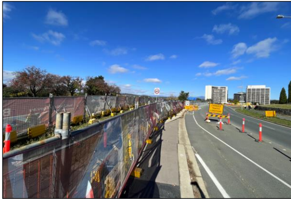
Photograph 22: Block 1 frontage to Vernon Circle with existing hoardings and temporary traffic management systems installed by Canberra Light Rail for raising London Circuit project.
