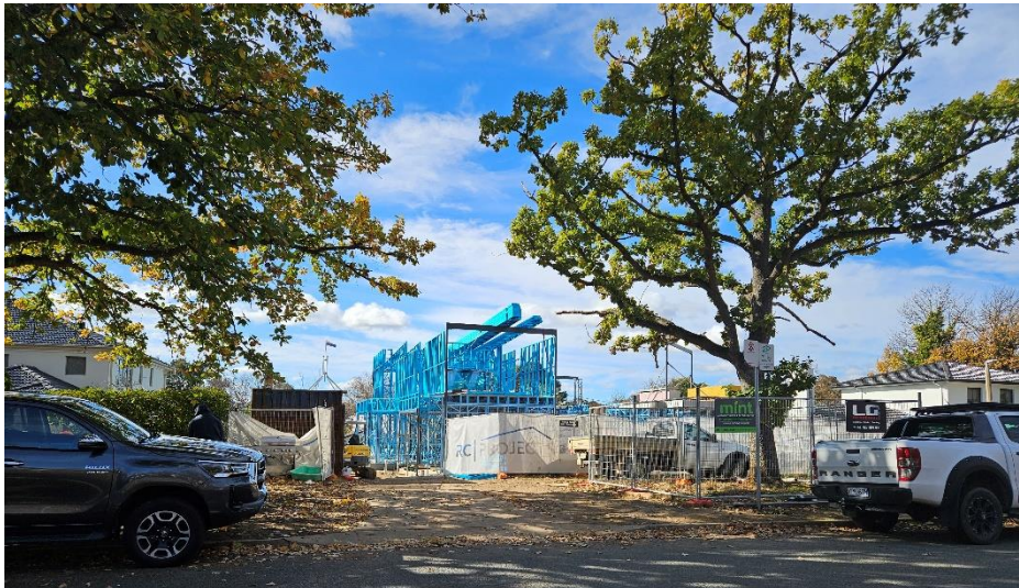
Pic 2 On going two storey re- development at Block 14 – 71 National Circuit. Modern Facade
