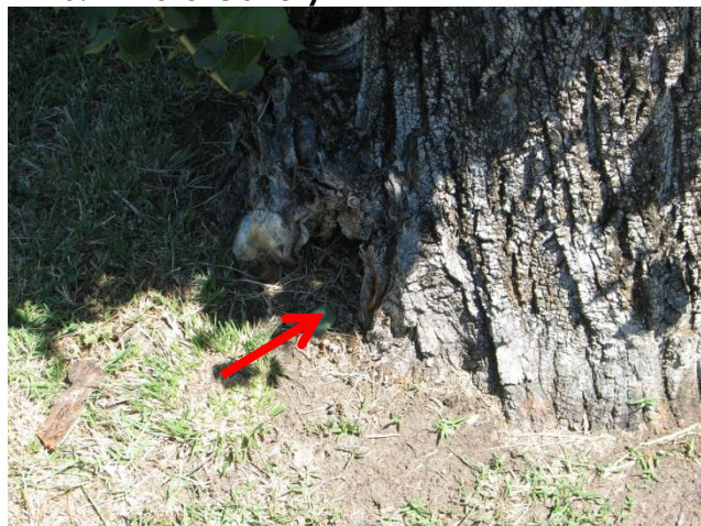
Figure 3 Decay has entered an old wound caused by mower impact. There are many new wounds in the trees from recent mower impact and whipper snipper use.
