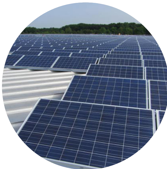
INTEGRATED SOLAR POWER
