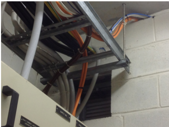
Photo No: J123625-003-CEN-787 Result: SMF - Positive Building/Level: Office Block-Basement Level Room/Location: Main Switch Room-Cables Feature/Material: Penetrations-Pillow Insulation
