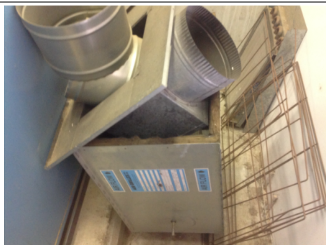
Photo No: J123625-003-CEN-767 Result: SMF - Positive Building/Level: Office Block-Level 3 Room/Location: Plant Room No.8-Redundant Plant Feature/Material: Duct-Insulation Material
