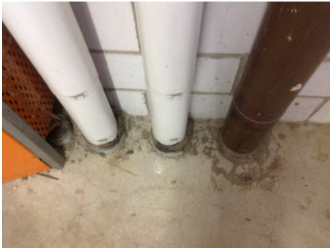
Photo No: J123625-003-CEN-773 Result: SMF - Positive Building/Level: Office Block-Level 2 Room/Location: Plant Rooms No.5 & No.6-Ceiling & floor - Pipes Feature/Material: Penetrations-Loose Insulation
