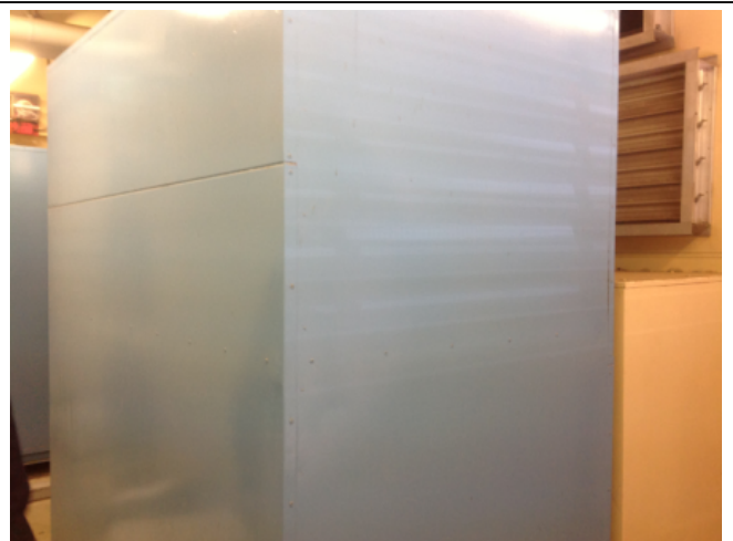
Photo No: J123625-003-CEN-771 Result: SMF - Positive Building/Level: Office Block-Level 2 Room/Location: Plant Rooms No.5 & No.6-AHU Feature/Material: Plant & Equipment-Insulation Material
