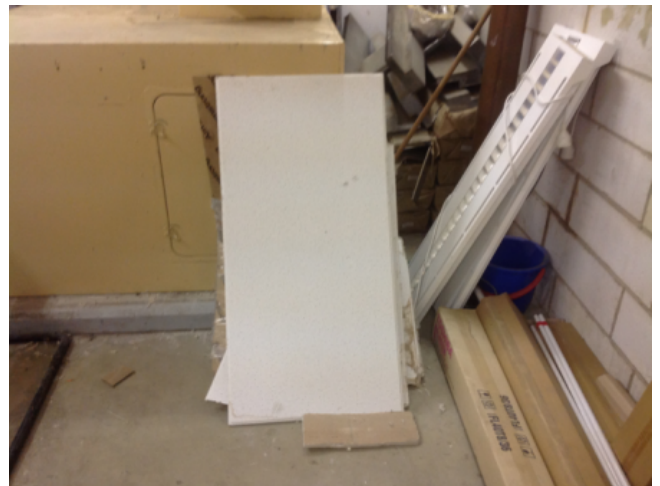
Photo No: J123625-003-CEN-786 Result: SMF - Positive Building/Level: Office Block-Ground Level Room/Location: Plant Room No.2- Feature/Material: Stored Item-Compressed Ceiling Tiles
