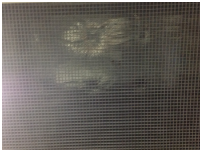
Photo No: J123625-003-CEN-766 Result: SMF - Positive Building/Level: Office Block-Level 3 Room/Location: Ceiling Space-Variou Throughout Feature/Material: Ductwork Insulation-Insulation Material
