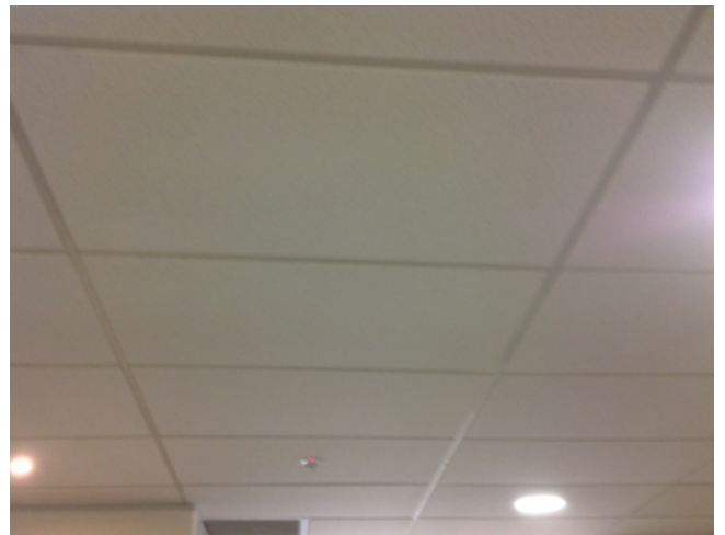
Photo No: J123625-003-CEN-765 Result: SMF - Positive Building/Level: Office Block-Level 3 Room/Location: Office Areas-Throughout Feature/Material: Ceiling Tiles-Compressed Ceiling Tiles
