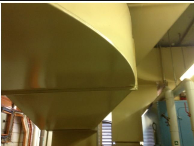
Photo No: J123625-003-CEN-778 Result: SMF - Positive Building/Level: Office Block-Level 1 Room/Location: Plant Rooms No.3 & No.4-A/C Feature/Material: Ductwork Insulation-Insulation Material
