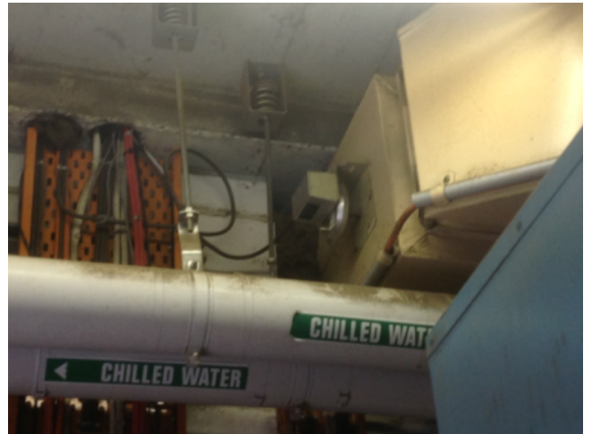
Photo No: J123625-003-CEN-774 Result: SMF - Positive Building/Level: Office Block-Level 2 Room/Location: Plant Rooms No.5 & No.6-Walls - Ductwork Feature/Material: Penetrations-Loose Insulation
