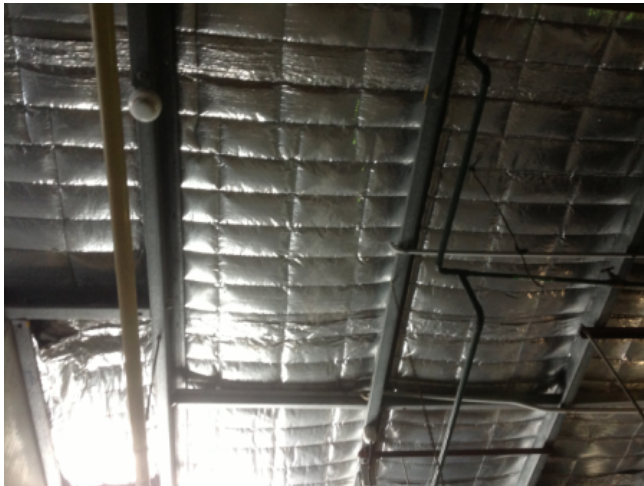
Photo No: J123625-003-CEN-755 Result: SMF - Positive Building/Level: Office Block-Level 4 Room/Location: All rooms-Throughout Feature/Material: Roof Lining-Sarking Insulation
