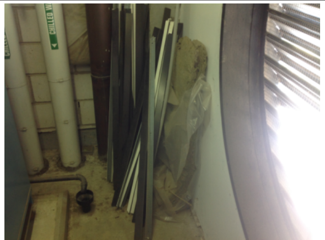
Photo No: J123625-003-CEN-768 Result: SMF - Positive Building/Level: Office Block-Level 3 Room/Location: Plant Room No.7-Loose Feature/Material: Stored Item-Insulation Material
