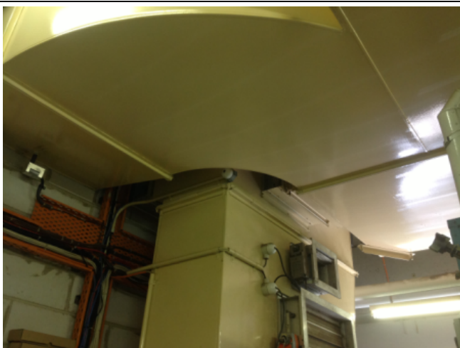
Photo No: J123625-003-CEN-772 Result: SMF - Positive Building/Level: Office Block-Level 2 Room/Location: Plant Rooms No.5 & No.6-A/C Feature/Material: Ductwork Insulation-Insulation Material
