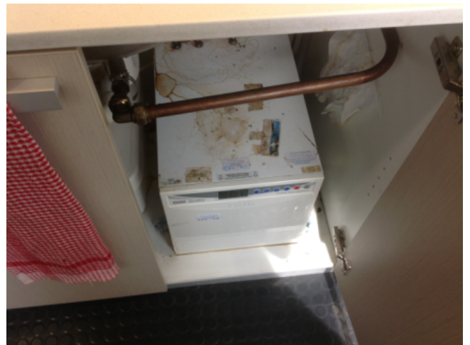
Photo No: J123625-003-CEN-780 Result: SMF - Positive Building/Level: Office Block-Level 1 Room/Location: Office Kitchens-Below sink Feature/Material: Hot Water Service Insulation-Insulation Material
