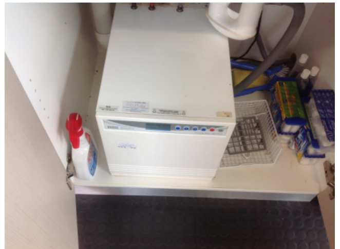
Photo No: J123625-003-CEN-775 Result: SMF - Positive Building/Level: Office Block-Level 2 Room/Location: Office Kitchens-Below sink Feature/Material: Hot Water Service Insulation-Insulation Material
