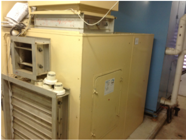
Photo No: J123625-003-CEN-763 Result: SMF - Positive Building/Level: Office Block-Level 3 Room/Location: Plant Rooms No.7 & No.8-AHU Feature/Material: Plant & Equipment-Insulation Material
