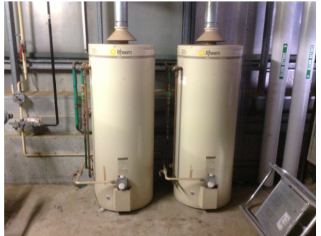
Photo No: J123625-003-CEN-756 Result: SMF - Positive Building/Level: Office Block-Level 4 Room/Location: Boiler Room- Feature/Material: Hot Water Service Insulation-Insulation Material
