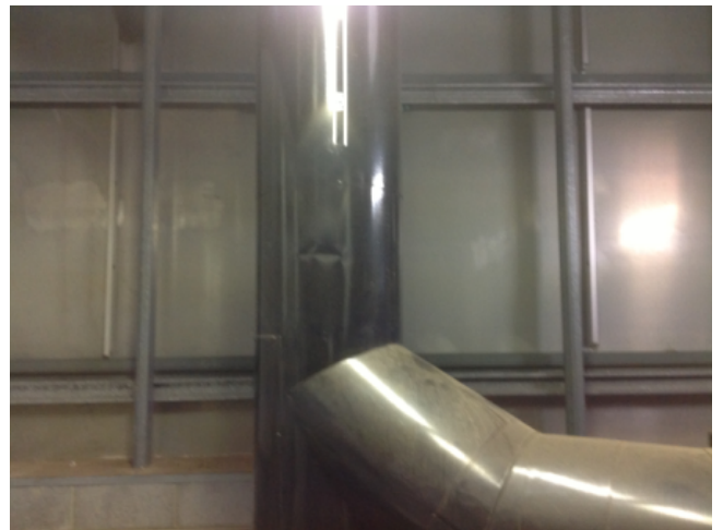
Photo No: J123625-003-CEN-758 Result: SMF - Positive Building/Level: Office Block-Level 4 Room/Location: Boiler Room-From boiler Feature/Material: Duct-Insulation Material
