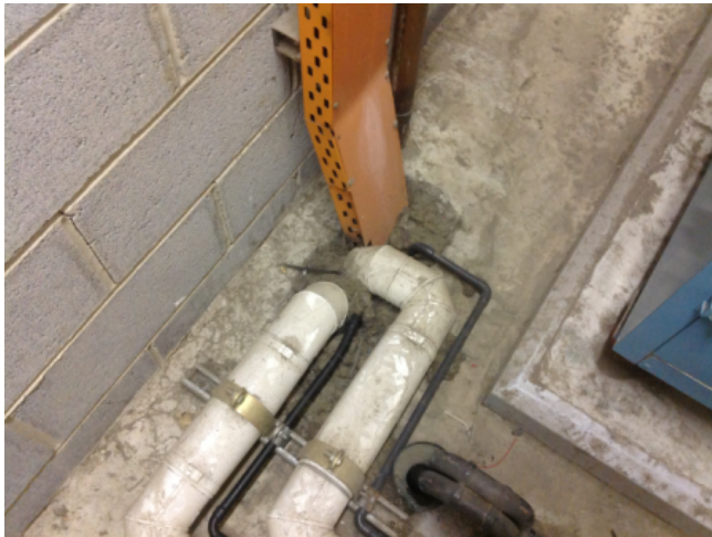
Photo No: J123625-003-CEN-781 Result: SMF - Positive Building/Level: Office Block-Ground Level Room/Location: Plant Rooms No.1 & No.2-Ceiling & floor - Pipes Feature/Material: Penetrations-Loose Insulation
