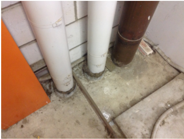
Photo No: J123625-003-CEN-776 Result: SMF - Positive Building/Level: Office Block-Level 1 Room/Location: Plant Rooms No.3 & No.4-Ceiling & floor - Pipes Feature/Material: Penetrations-Loose Insulation
