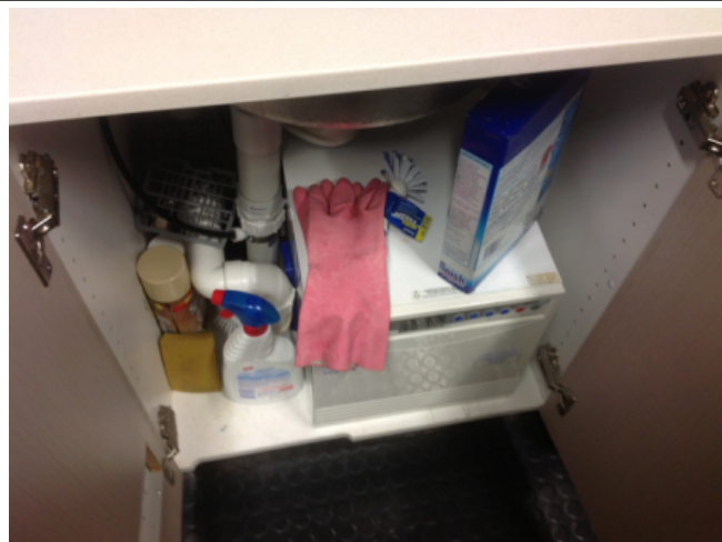
Photo No: J123625-003-CEN-769 Result: SMF - Positive Building/Level: Office Block-Level 3 Room/Location: Office Kitchens-Below sink Feature/Material: Hot Water Service Insulation-Insulation Material
