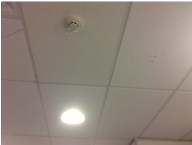
Photo No: J123625-003-CEN-770 Result: SMF - Positive Building/Level: Office Block-Level 2 Room/Location: Office Areas-Throughout Feature/Material: Ceiling Tiles-Compressed Ceiling Tiles
