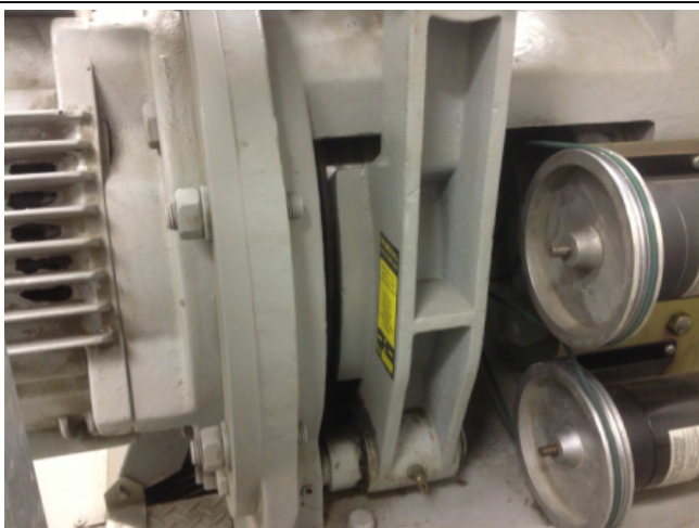
Photo No: J123625-003-CEN-754 Result: Asbestos - Presumed Positive Building/Level: Office Block-Level 4 Room/Location: Lift Motor Room-Lift No.'s 1 & 2 Feature/Material: Lift Motor-Brake Pads
