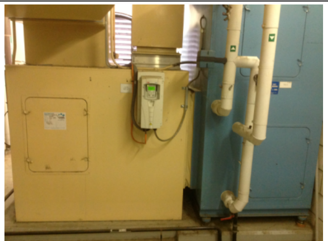
Photo No: J123625-003-CEN-777 Result: SMF - Positive Building/Level: Office Block-Level 1 Room/Location: Plant Rooms No.3 & No.4-AHU Feature/Material: Plant & Equipment-Insulation Material
