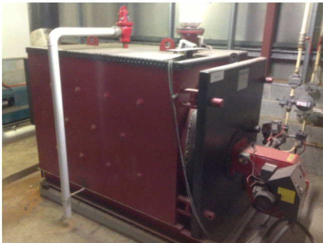
Photo No: J123625-003-CEN-757 Result: SMF - Positive Building/Level: Office Block-Level 4 Room/Location: Boiler Room-Central Feature/Material: Plant & Equipment-Insulation Material
