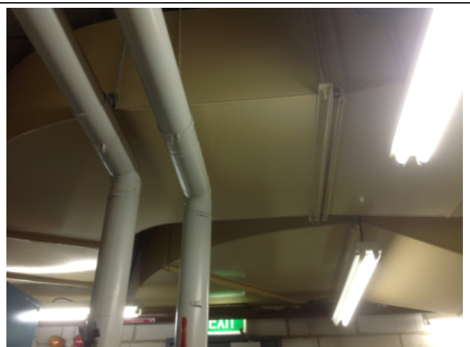
Photo No: J123625-003-CEN-764 Result: SMF - Positive Building/Level: Office Block-Level 3 Room/Location: Plant Rooms No.7 & No.8-A/C Feature/Material: Ductwork Insulation-Insulation Material
