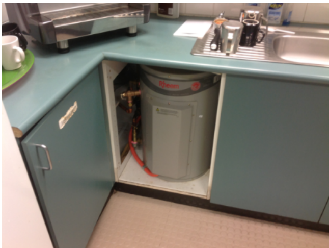
Photo No: J123625-003-CEN-785 Result: SMF - Positive Building/Level: Office Block-Ground Level Room/Location: Office Kitchens-Below sink Feature/Material: Hot Water Service Insulation-Insulation Material
