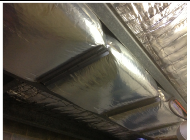
Photo No: J123625-003-CEN-760 Result: SMF - Positive Building/Level: Office Block-Level 4 Room/Location: Plant Rooms-Variou Throughout Feature/Material: Ductwork Insulation-Insulation Material
