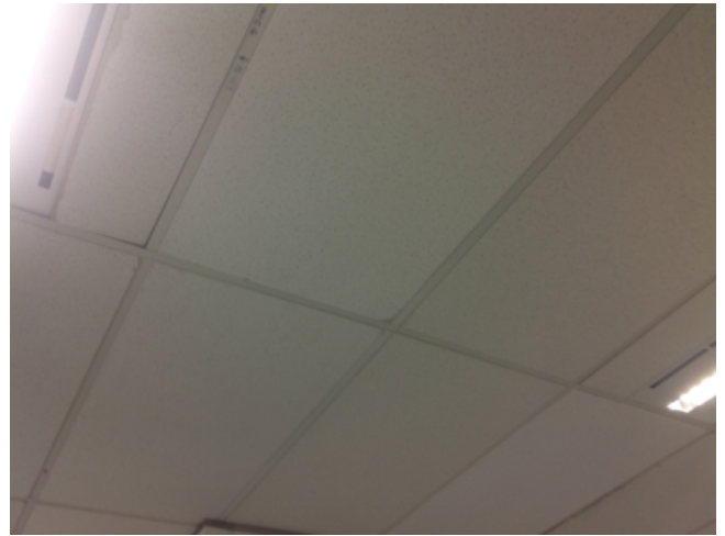
Photo No: J123625-003-CEN-784 Result: SMF - Positive Building/Level: Office Block-Ground Level Room/Location: Office Areas-Throughout Feature/Material: Ceiling Tiles-Compressed Ceiling Tiles
