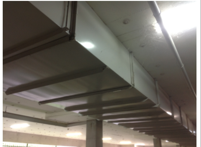
Photo No: J123625-003-CEN-788 Result: SMF - Positive Building/Level: Office Block-Basement Level Room/Location: Car Park-A/C Feature/Material: Ductwork Insulation-Insulation Material
