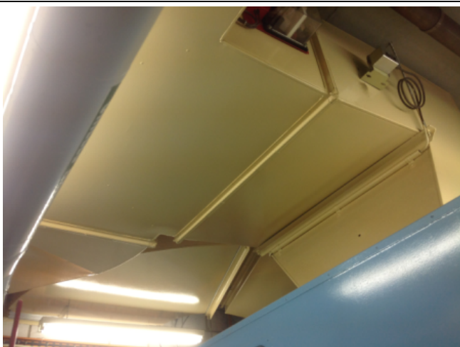
Photo No: J123625-003-CEN-783 Result: SMF - Positive Building/Level: Office Block-Ground Level Room/Location: Plant Rooms No.1 & No.2-A/C Feature/Material: Ductwork Insulation-Insulation Material
