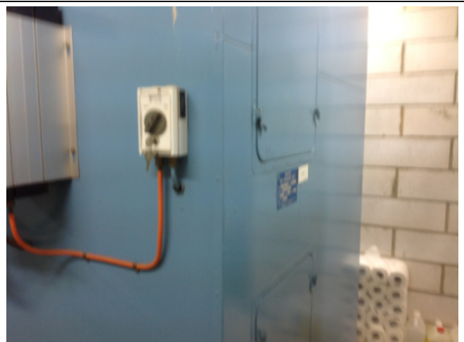
Photo No: J123625-003-CEN-782 Result: SMF - Positive Building/Level: Office Block-Ground Level Room/Location: Plant Rooms No.1 & No.2-AHU Feature/Material: Plant & Equipment-Insulation Material
