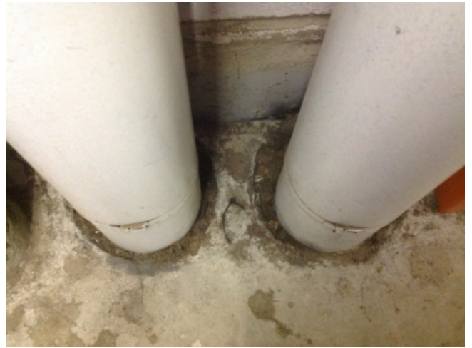
Photo No: J123625-003-CEN-761 Result: SMF - Positive Building/Level: Office Block-Level 3 Room/Location: Plant Rooms No.7 & No.8-Ceiling & floor - Pipes Feature/Material: Penetrations-Loose Insulation
