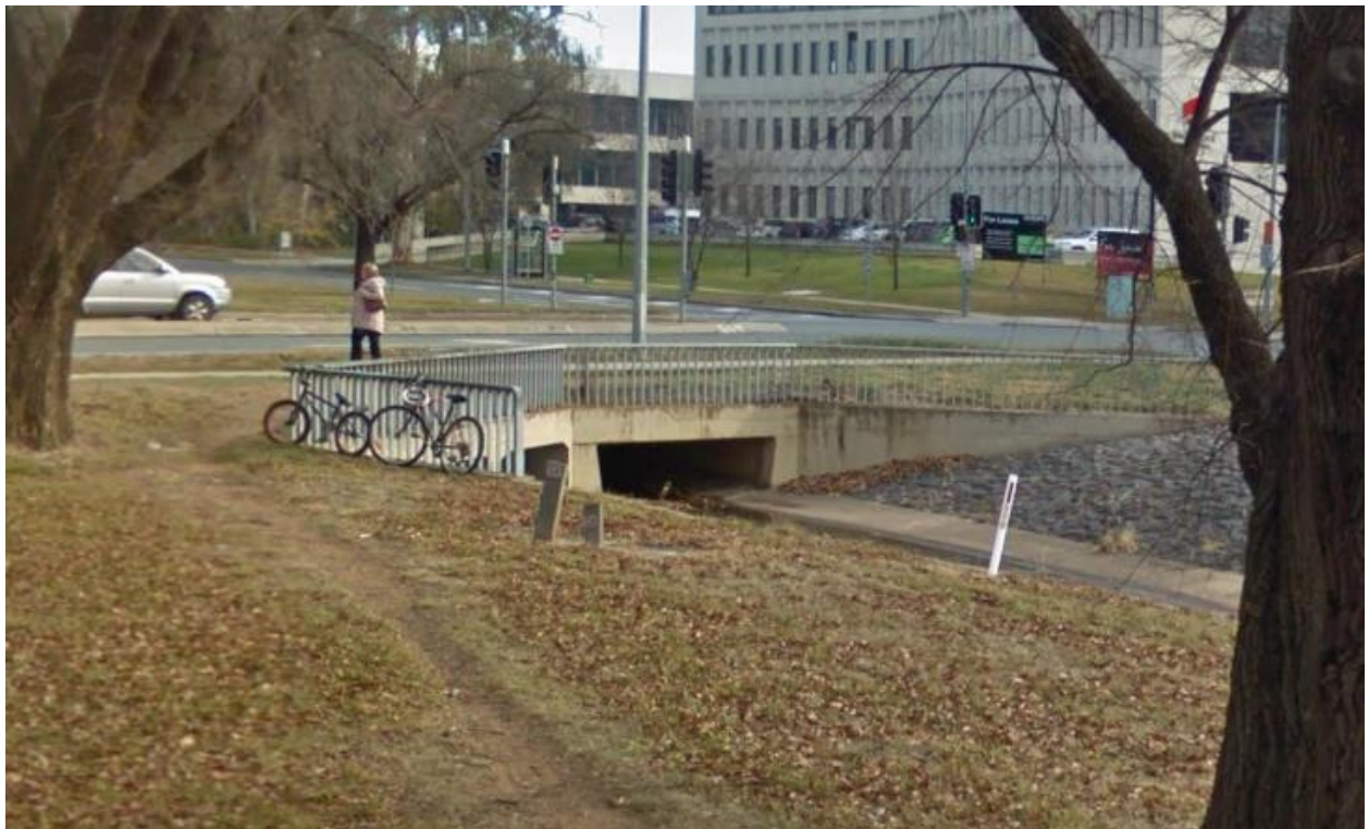
Figure 2 – Box culvert outlet into Concrete lined channel in median of Brisbane Avenue
