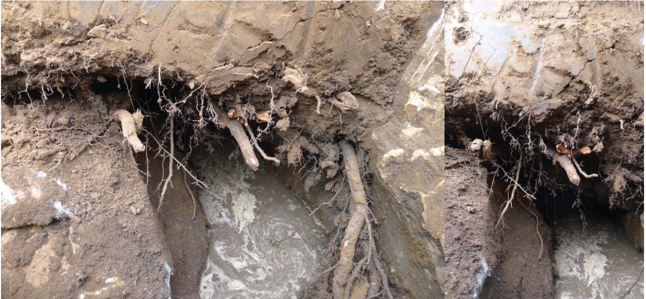
Figure 4 - Root network and void within Trial Pit 2
